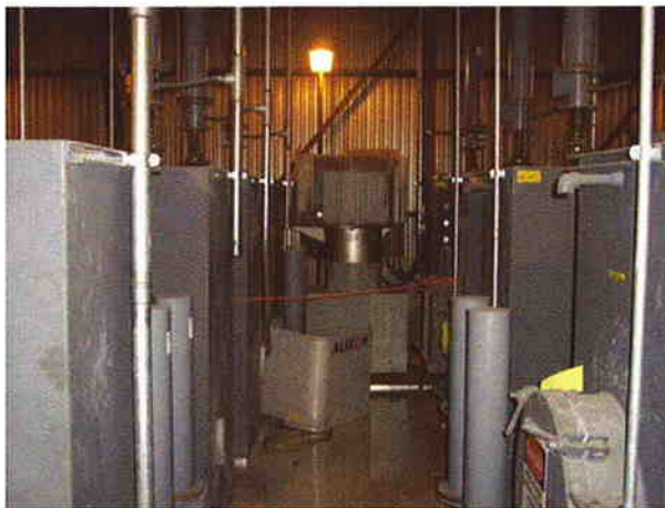
Nooter Construction Company recently completed electrostatic precipitator upgrades at Detroit Edison's Monroe Power Plant – one of the largest coal-burning power plants in the nation.
